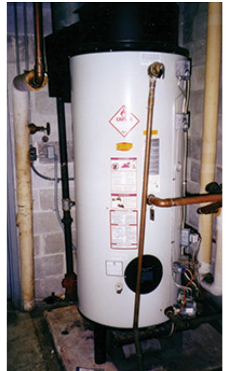
Figure 10. A T&P valve protecting the water heater
